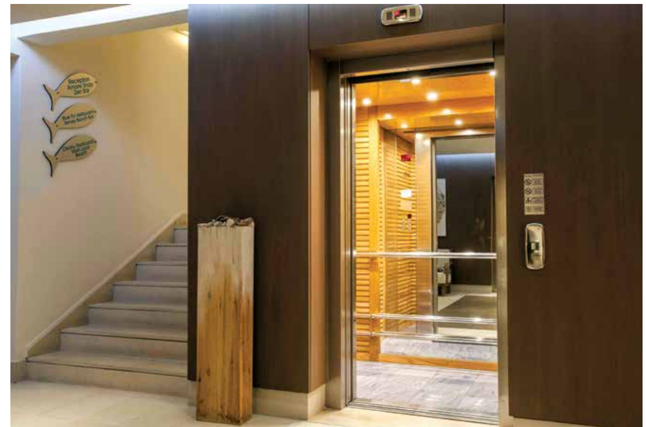
| Hydraulic Passenger lift (HAI)
